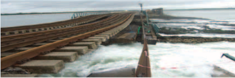
On 21 August 2009 the Broadmeadow Viaduct at Malahide collapsed, causing a three month closure of the Dublin-Drogheda section of the Dublin-Belfast line. A Railway Safety Commission investigation found four serious cases of non-compliance with rail safety regulations.
